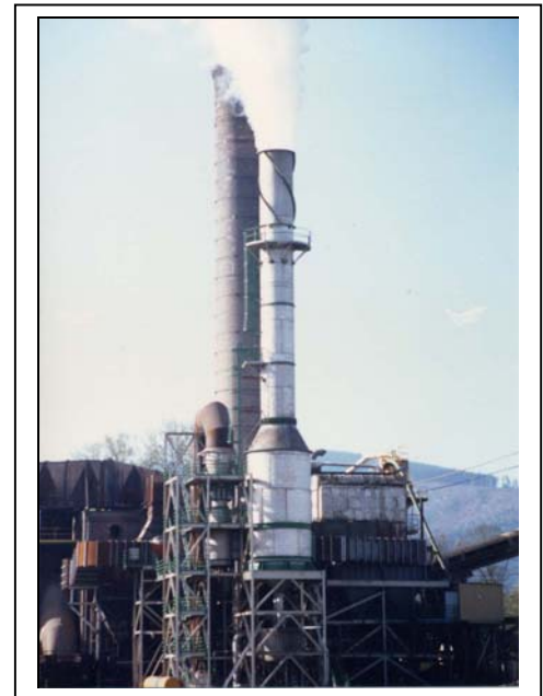
VENTURI SCRUBBER INSTALLED ON POWER BOILER
